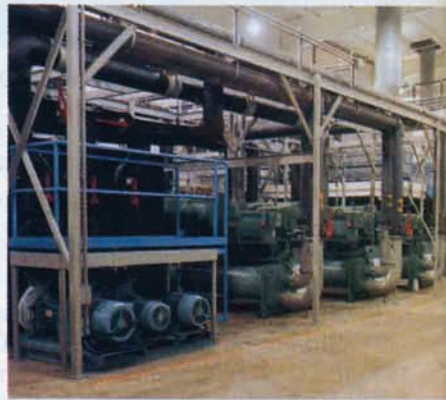
▲ A wastewater neutralization section, duplex deionized water system and acid purification unit are key to the waste treatment process.
